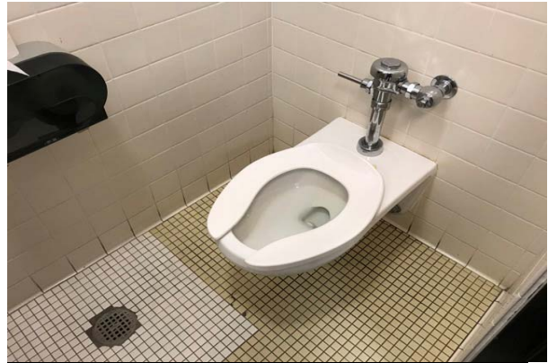
#20: TOILET, TANKLESS (WATER CLOSET)
