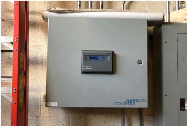
#37: BUILDING AUTOMATION SYSTEM (HVAC CONTROLS)
