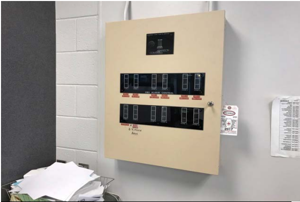
#49: FIRE ALARM CONTROL PANEL, ADDRESSABLE
