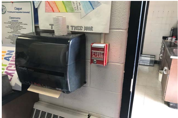
#40: FIRE ALARM DEVICE
