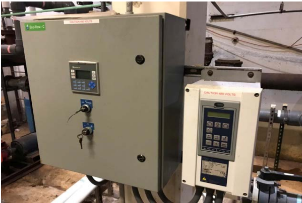
#45: VARIABLE FREQUENCY DRIVE (VFD)
