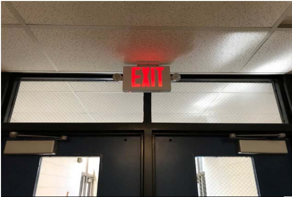
#43: EXIT LIGHTING FIXTURE
