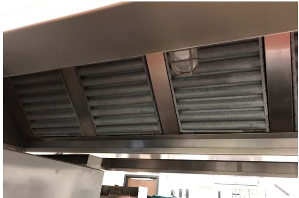
#52: COMMERCIAL KITCHEN, EXHAUST HOOD
