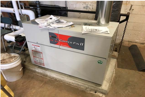
#21: SWIMMING POOL HEATER, GAS-FIRED
