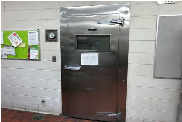
#51: COMMERCIAL KITCHEN, WALK-IN REFRIGERATOR
