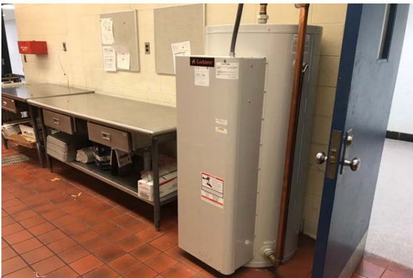
#23: WATER HEATER, ELECTRIC
