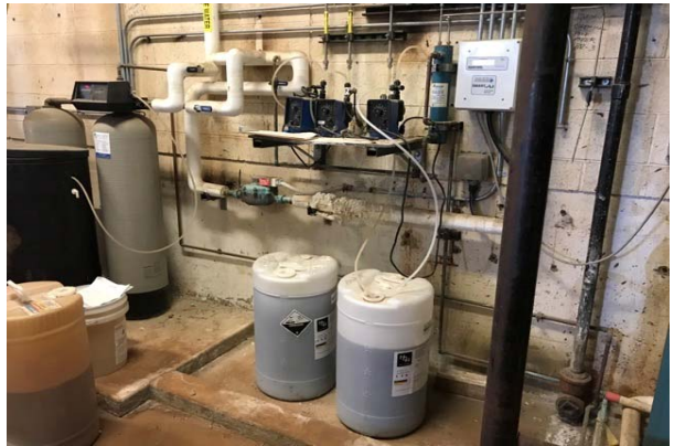
#34: CHEMICAL FEED SYSTEM
