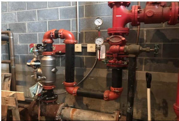
#47: EXISTING SPRINKLER SYSTEM
