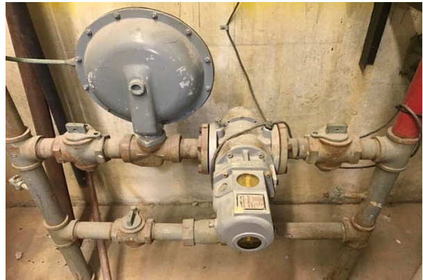
#46: NATURAL GAS REGULATOR/METER
