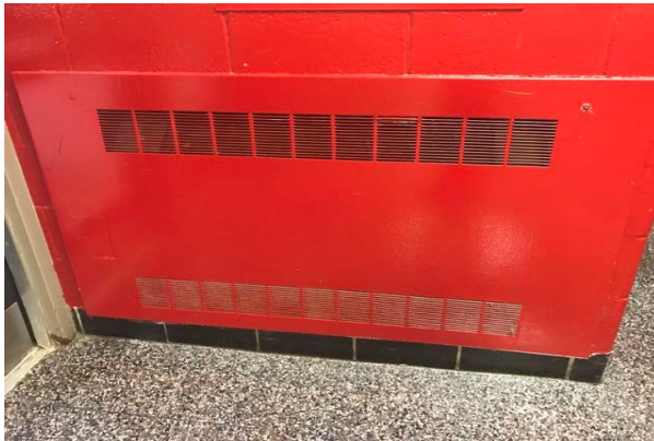
#45: RADIATOR, HYDRONIC CABINET
