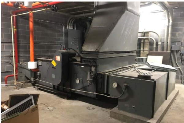
#41: AIR HANDLER, ORIGINAL
