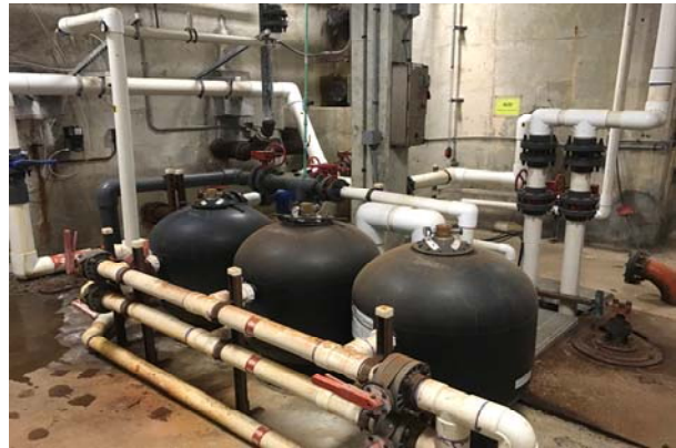
#40: SWIMMING POOL EQUIPMENT
