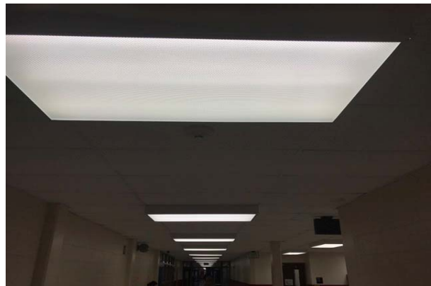
#54: T-8 LIGHTING SYSTEM
