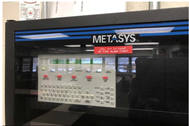
#48: FIRE ALARM PANEL
