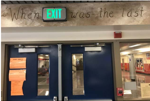
#49: FIRE SAFETY COMPONENTS
