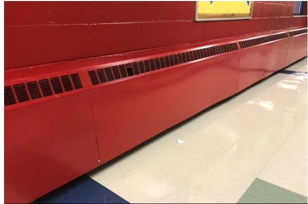
#44: RADIATOR, HYDRONIC BASEBOARD
