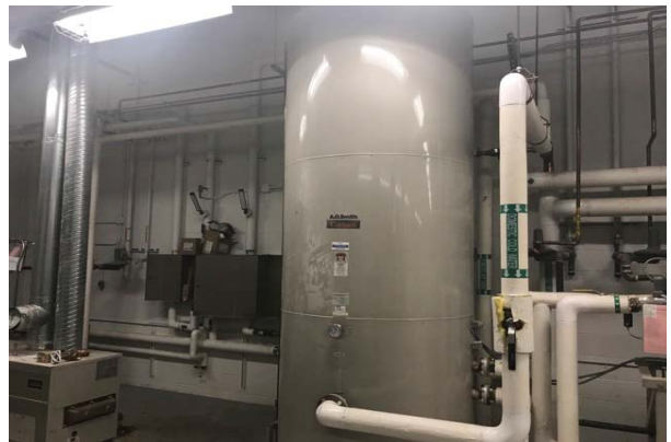
#34: WATER STORAGE TANK
