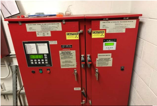
#55: FIRE PUMP CONTROLLER
