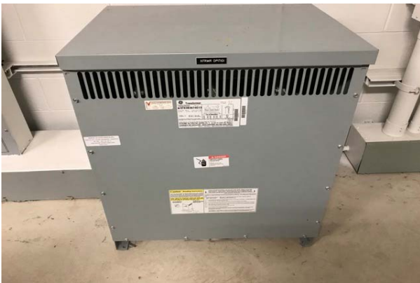
#47: STEP DOWN TRANSFORMER
