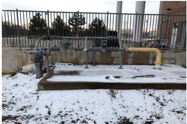
#40: NATURAL GAS SERVICE
