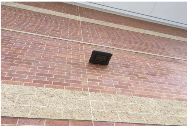
#15: EXTERIOR BUILDING LIGHTING
