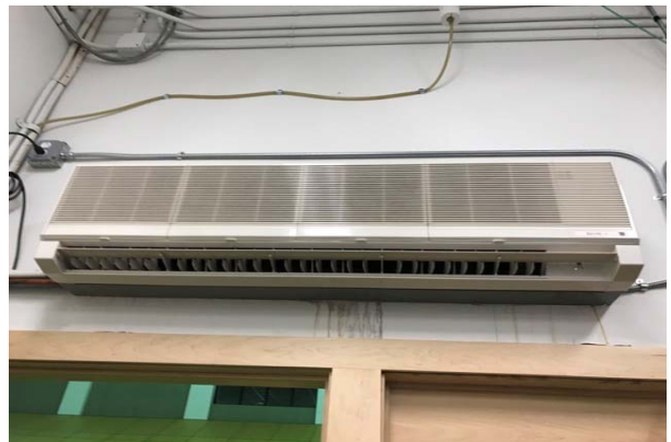
#30: DUCTLESS SPLIT SYSTEM
